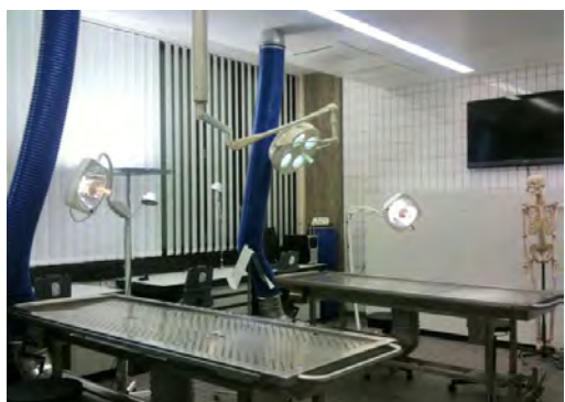
New infrastructure such as fully ventilated dissection tables
